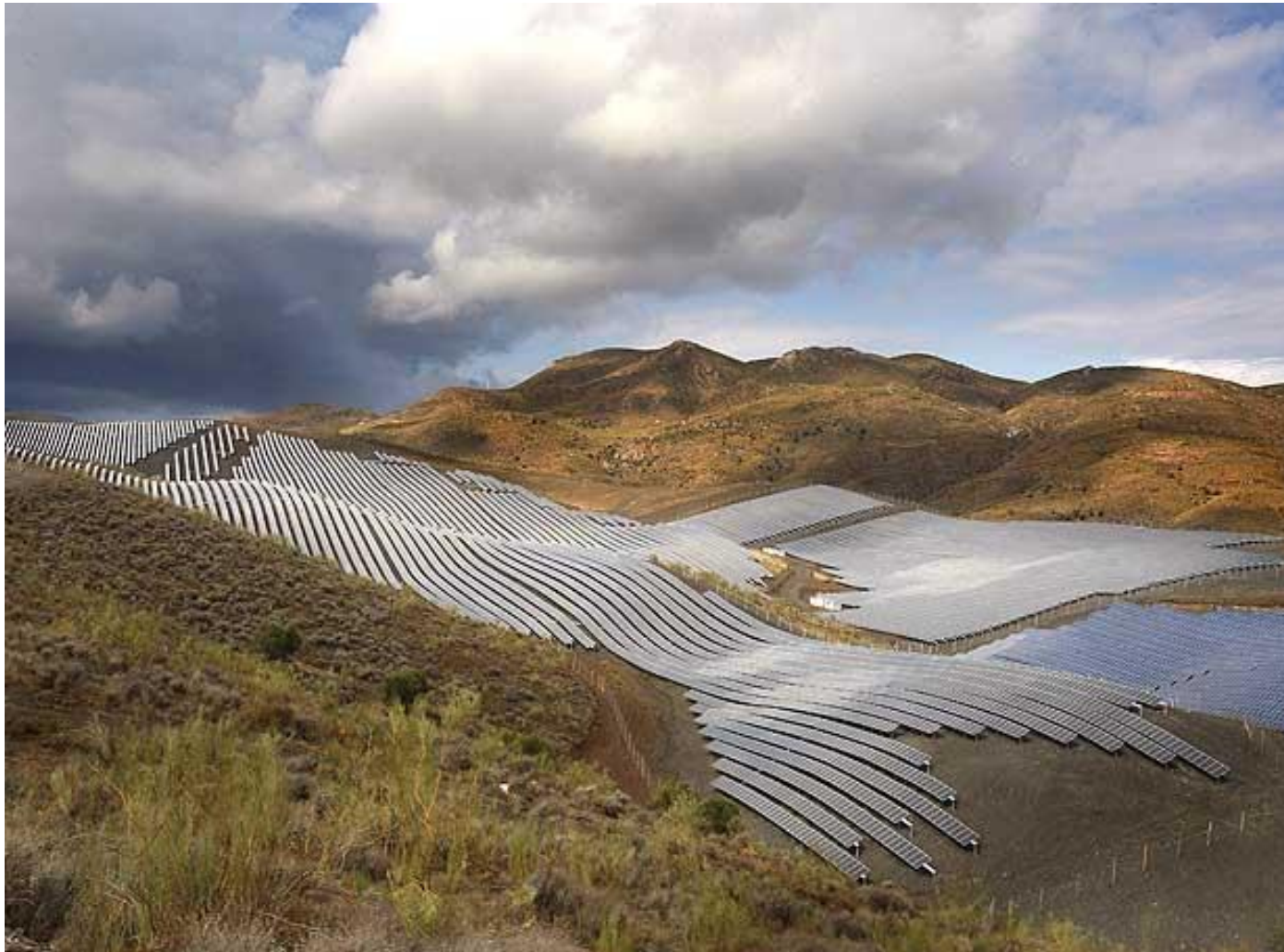
Grid-connected solar PV power plant. 21 MW
